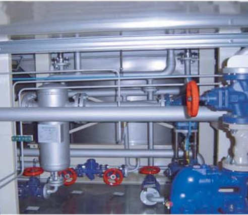
Heat Exchanger Tightness Control
