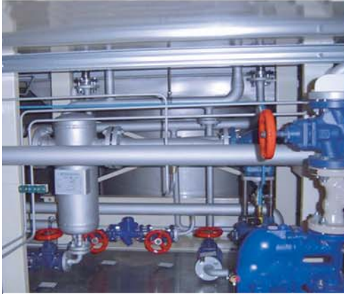
Heat Exchanger Tightness Control
